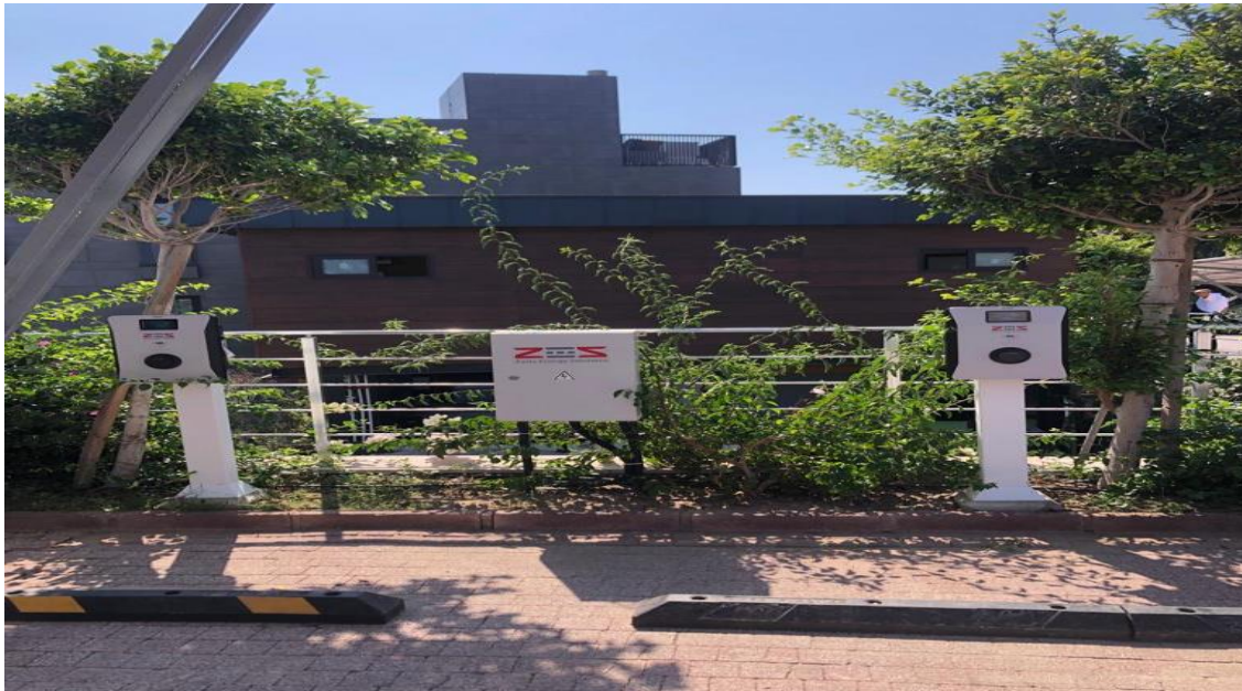
Electric Vehicle Charging Station
