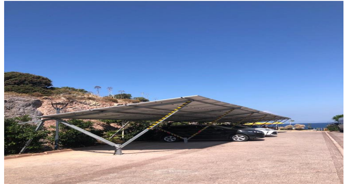
Solar Energy System
