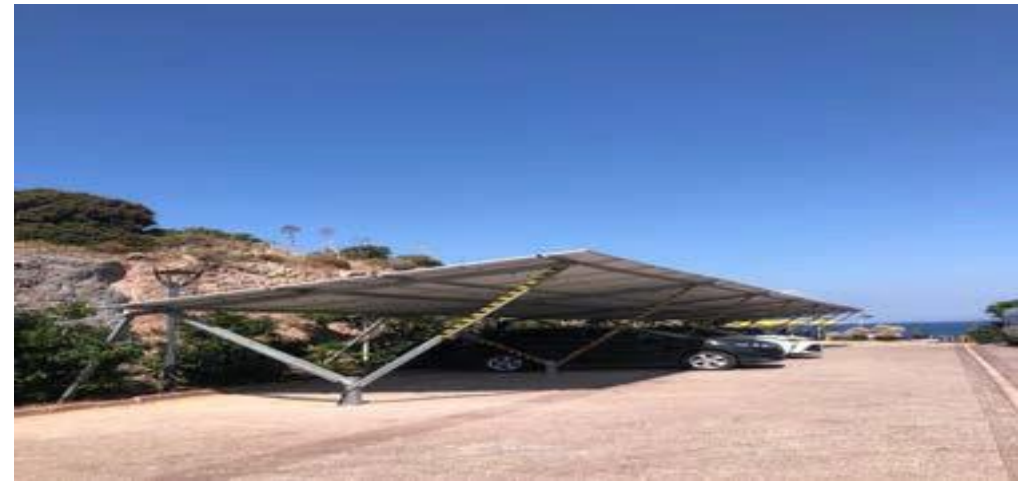
Solar Energy System
