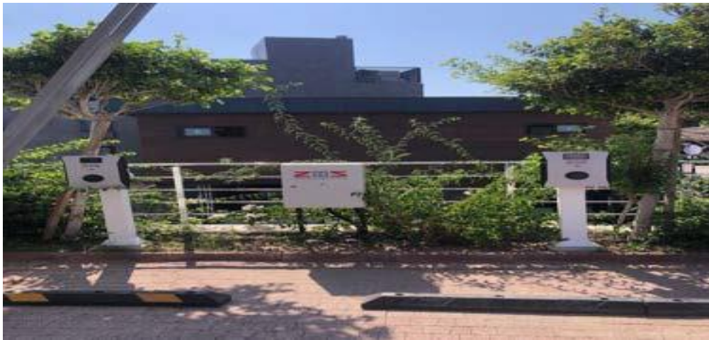
Electric Vehicle Charging Station
